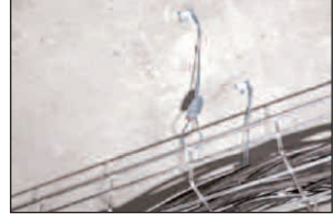
Light weight Cable Trays / Lights
